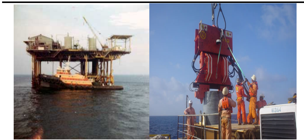
Figure 4.14 Construction of Piled Marine Platform for use in Bored Piling works in open sea conditions
