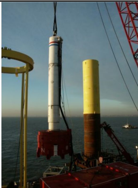
Figure 4.12 Installation of Monopile Turbine Foundation at 60MW Scroby Sands Wind Farm, UK (Source: http://www.mammoetvanoord.com/webfront/base.asp?pageid=26 )
