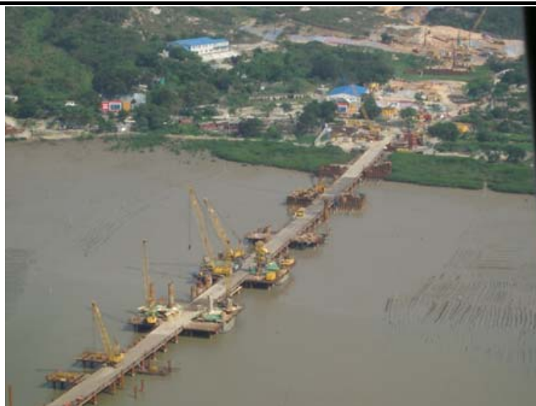
Figure 4.13 Construction of Temporary Access Bridge in Deep Bay for the Hong Kong - Shenzhen Western Corridor/Deep Bay Link
